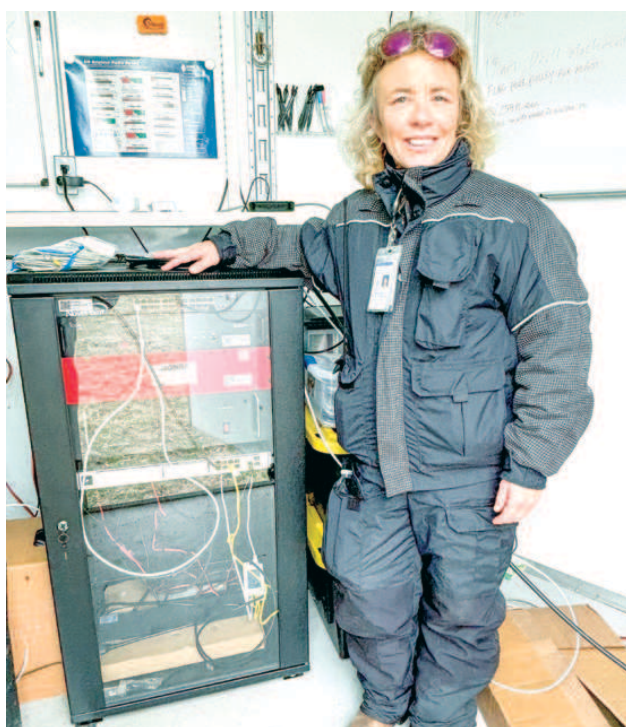
NEWEST ADDITION -- Lee County ARES Emergency Coordinator Marida Favia del Core Borromeo stands next to a brand new Repeater device recently installed in the ARES trailer. The Repeater picks up local radio signals and rebroadcasts them on different frequencies at a much further distance. On a high vantage point, a signal could be boosted 20 to 30 miles.
